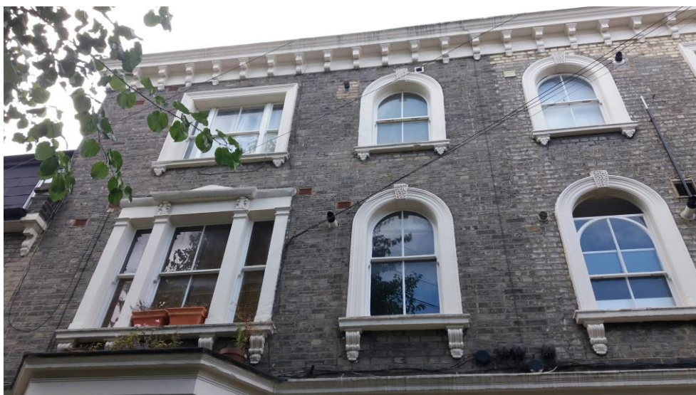
Deep cornices with moulded modillions. An original feature of nos. 2-10 Barclay Road. Missing on 2 & 4.
